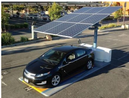
Fig.no. 2: Stand-alone PV energy Electric battery vehicle charging station .
